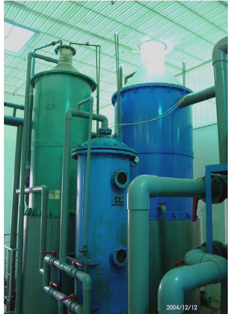
parallel connection of foam separator
